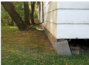
This foundation wall for Cabin E and F is falling. We need to rebuild the foundation of this cabin.
